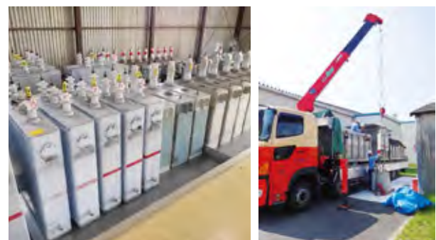
PCB-containing equipment being transported to JESCO
